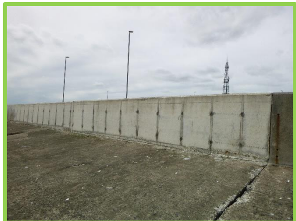
Section of recently replaced rear wall. (Asset Ref. No. 121AB901B0802C01)
