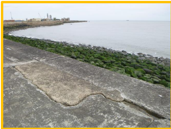
Damaged cope blocks and deck slab (Asset Ref. 121AB901B0802C02)
