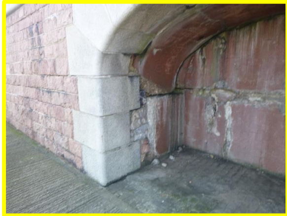
Damage in upper wall recess. (Asset Ref. No. 121AB901B0703C01)
