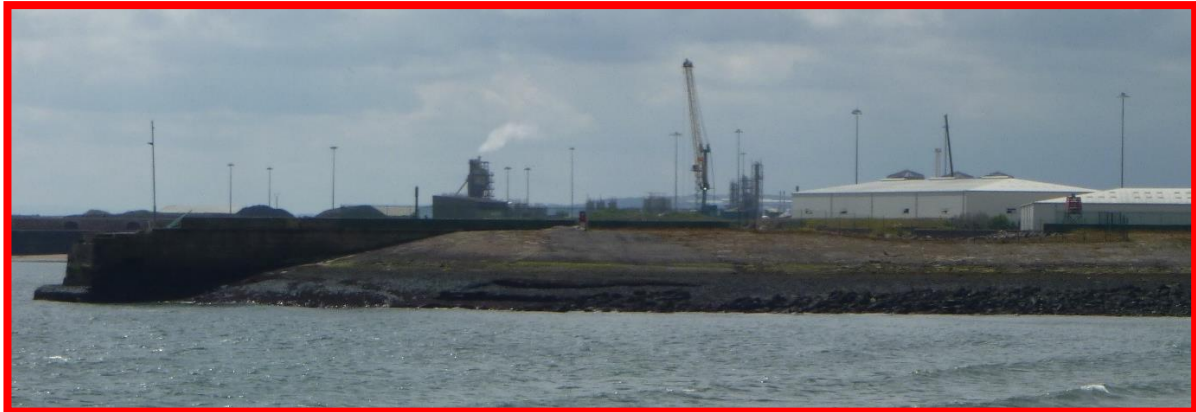
Northern face of Old North Pier, voids at toe (Asset Ref. No. 121AB901B0702C03)
