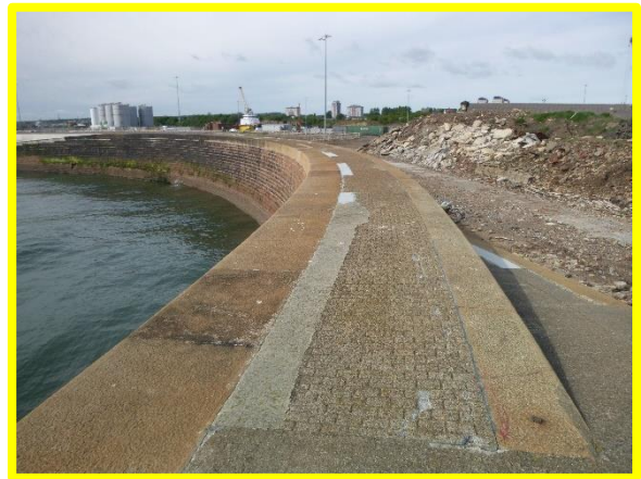
Local repairs to upper deck from root of pier. (Asset Ref. No. 121AB901B0703C01)
