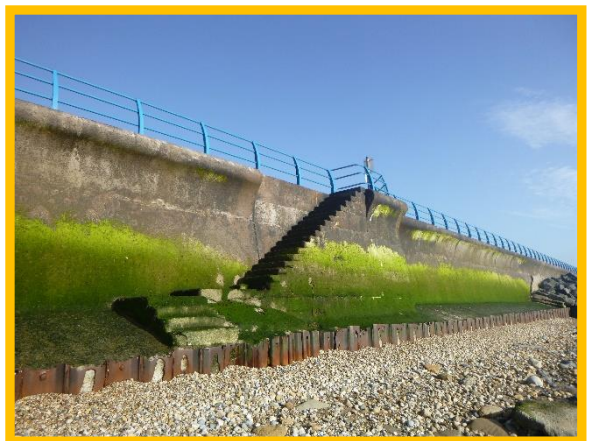
Exposed reinforcement to seawall and redundant steps. (Asset Ref. No. 121AB901B0803C02)
