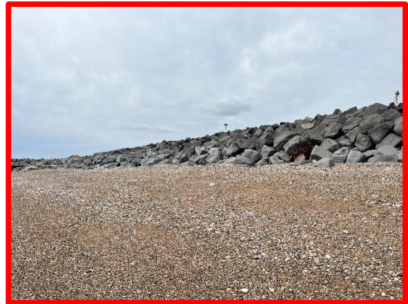
Derelict concrete groyne from south. (Asset Ref. No. 121AB901B0801C06)
