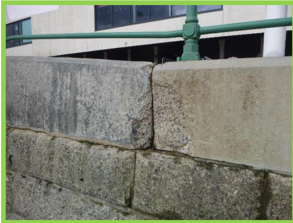
Localised damage on repaired section of coping. (Asset Ref No. 121AB901B0603C01)
