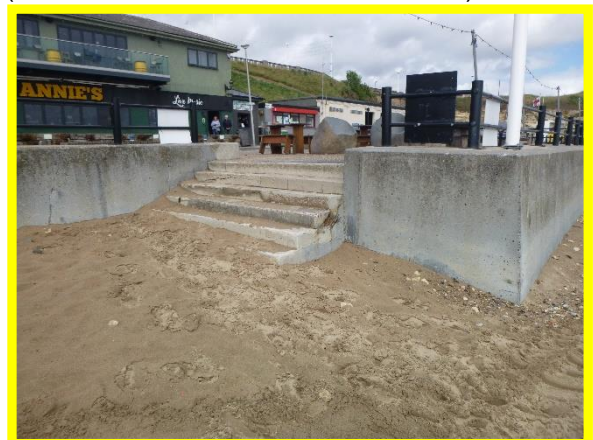
Southern access steps in fair condition with historic repair holding. (Asset Ref. No. 121AB901B0605C02)
