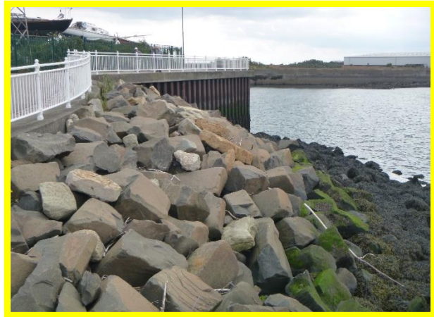
Sheet piling at "Rat House Corner" in fair condition (Asset Ref. 121AB901B0702C03)
