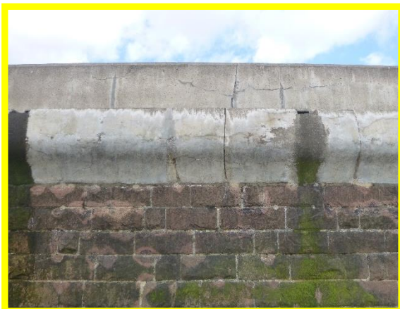
Cracking in seaward side of crest wall (Asset Ref. No. 121AB901B0603C03)
