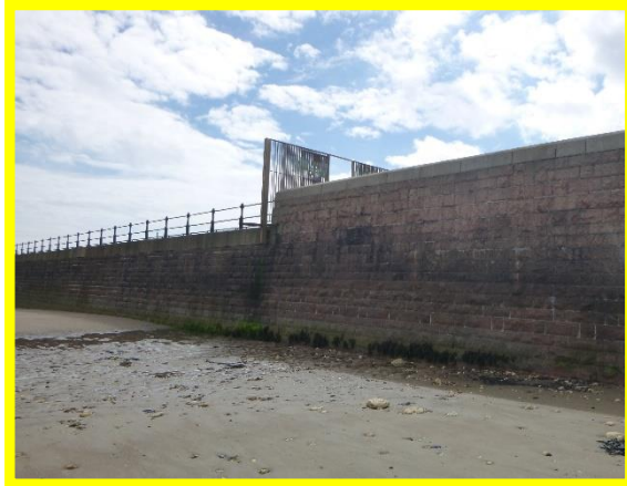
View on northern side of masonry wall at root of pier – localised abrasion and mortar loss. (Asset Ref. No. 121AB901B0702C05)
