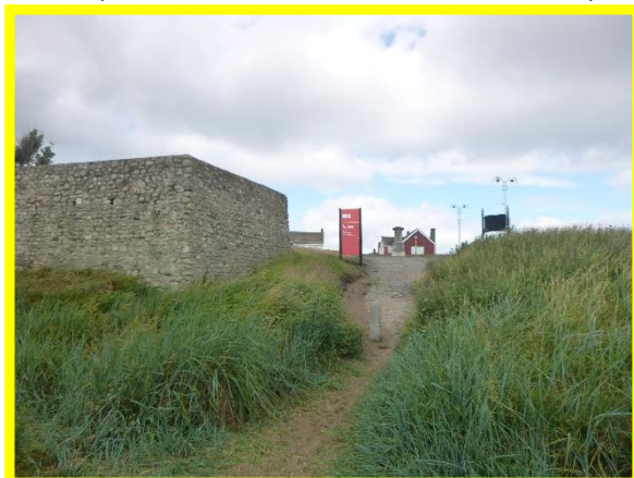
Access ramp at Whitburn Steel, toe undercut during previous inspections. (Asset Ref No. 121AB901B0602C01)
