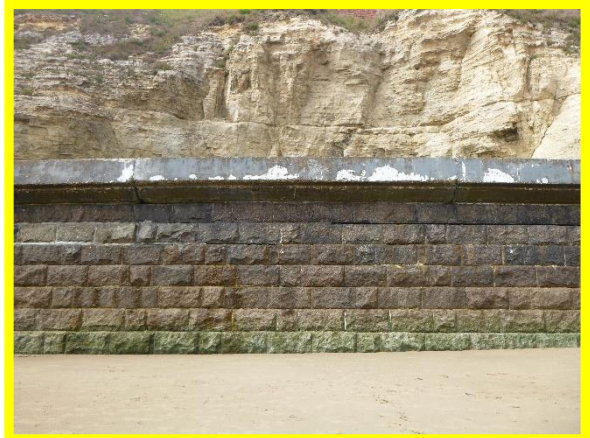
Area of missing blocks repaired since 2018, part of longitudinal crack remains. (Asset Ref. No. 121AB901B0605C01)
