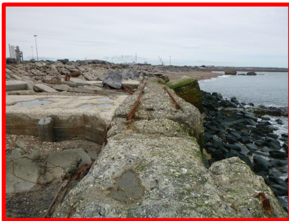
Buttress detached from main structure and heavily abraded deck (Asset Ref. No. 121B901B0801C07)
