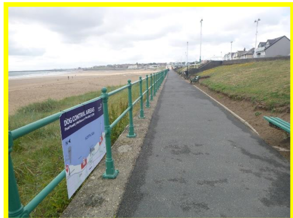
Asphalt surface appears in good condition, erosion to rear embankment (Asset Ref No. 121AB901B0603C01)
