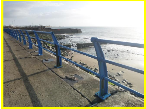
Localised section of damaged railing (Asset Ref. No. 121AB901B0803C02).
