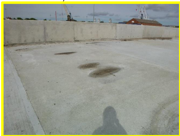
Depressions in deck slab. (Asset Ref. No. B901B0801C03)
