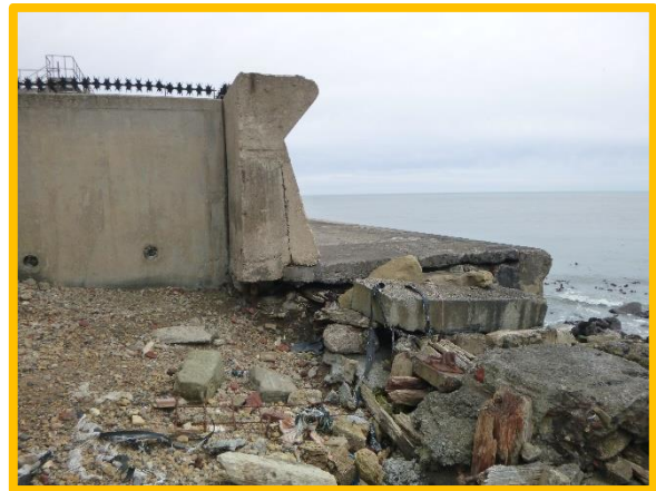
Undermining of upper seawall at south end. (Asset Ref. No. 121AB901B0802C04)
