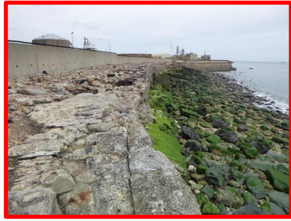
Rock armour in poor condition similar to previous inspections. (Asset Ref. No. 121B901B0802C03)
