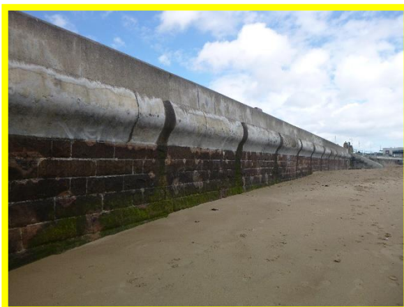
Several open joints in wall, beach levels the same as in 2020 with previously exposed voids buried. (Asset Ref. No. 121AB901B0603C03)
