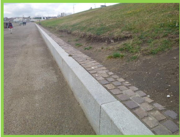
Erosion along the crest of the low retaining wall at the rear of the promenade. (Asset Ref No. 121AB901B0603C01)
