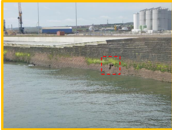
Localised missing blocks worsened (since 2020) and open joint, similar(to 2020). (Asset Ref. No. B901B0801C03)
