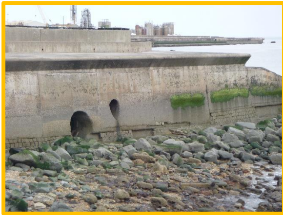
Missing facing masonry requires attention. (Asset Ref. No. 121AB901B0802C01)
