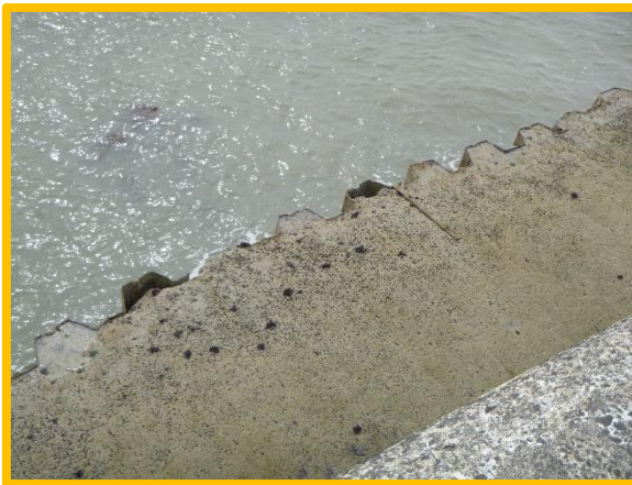
Corroded/abraded sheet pile wall at toe. (Asset Ref. No. 121AB901B0802C04)
