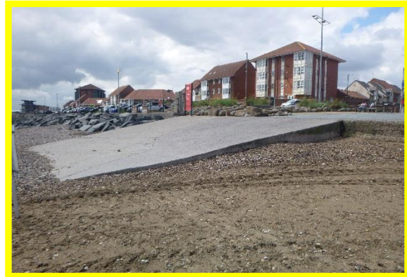
Slipway at southern end of wall in fair condition. (Asset Ref. No. 121AB901B0702C01)
