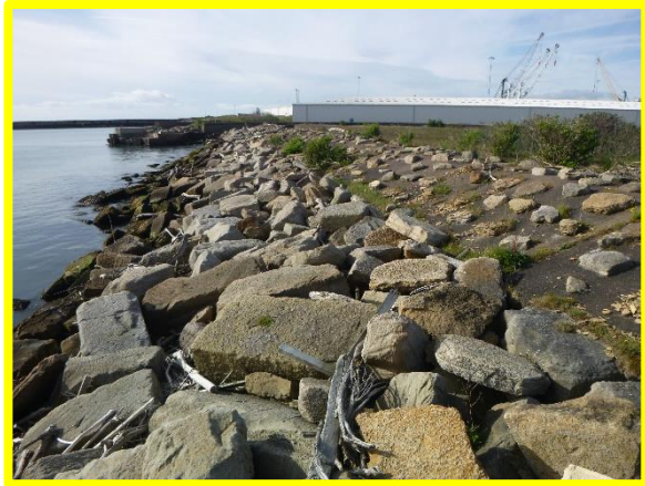
View of rock revetment from north showing loosely placed armour (Asset Ref. No. 121AB901BO703C03)
