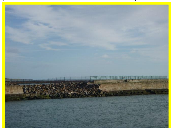
Old North Pier southern face showing extent of the breach. (Asset Ref. No. 121AB901B0702C03)
