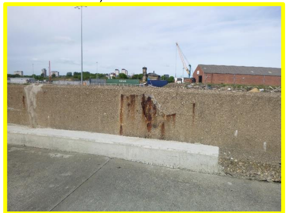
Remaining section of original splash wall in poor condition. (Asset Ref. No. B901B0801C03)
