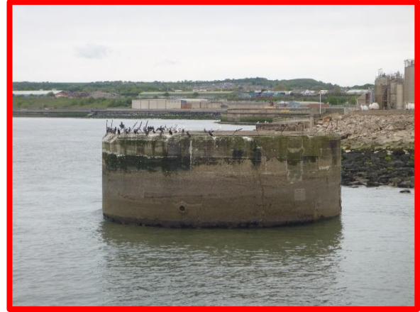
The roundhead is undercut, and the deck is heavily abraded. (Asset Ref. 121AB901B0802C05)
