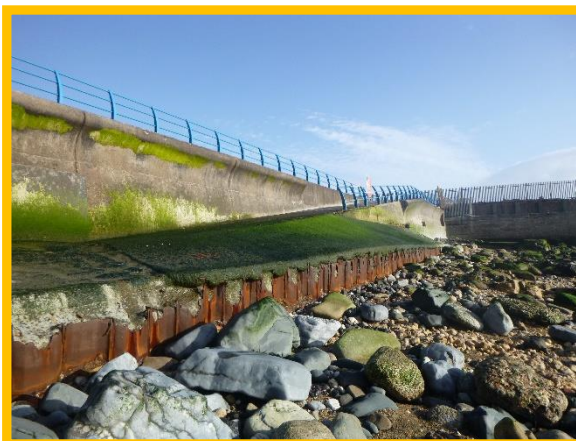
Heavily abraded and corroded steel toe piling (northernmost slipway). (Asset Ref. No. 121AB901B0803C02)
