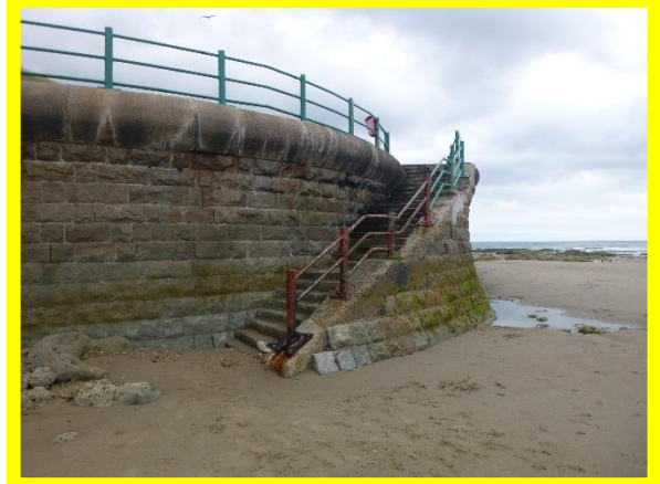
Access steps at southern end of defence in fair condition. (Asset Ref. No. 121AB901B0604C02)
