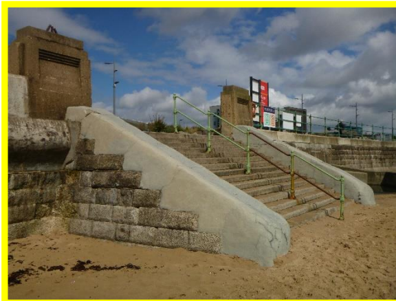
Repairs to step abutments in fair condition. Handrail is corroded in places (Asset Ref No. 121AB901B0603C02)
