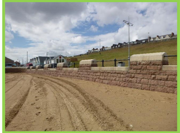
Southern section of masonry wall protected by wide beach in good overall condition. (Asset Ref. No. 121AB901B0605C02)
