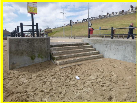
Northern access steps in fair to poor condition requiring minor repairs. (Asset Ref. No. 121AB901B0605C02)
