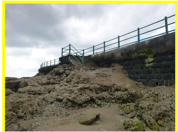
Eroded natural rock at access steps to Parsons Rocks (access to steps blocked by handrail). (Asset Ref. No. 121AB901B0604C02)
