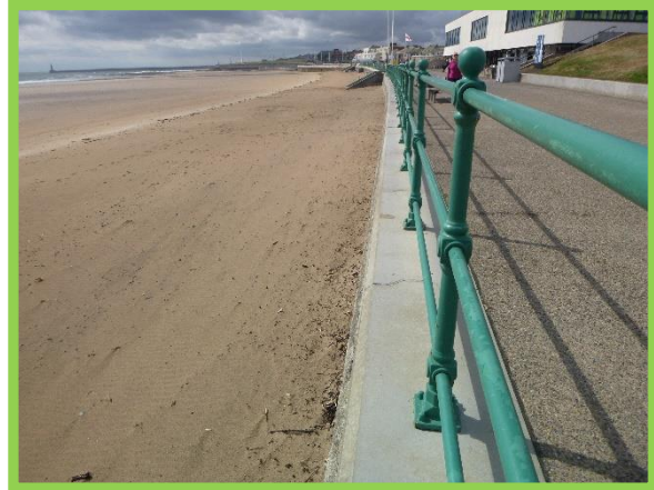
Repaired section of coping blocks in good condition. (Asset Ref No. 121AB901B0603C01)
