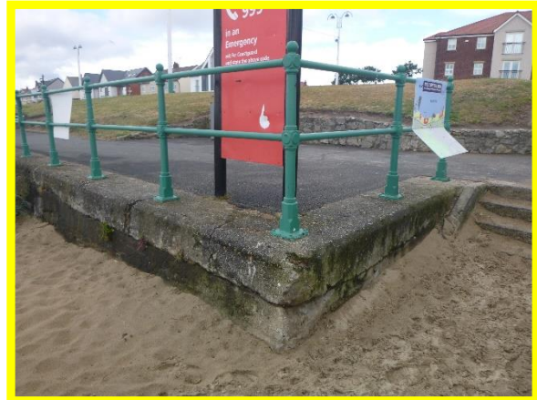
Spalled/damaged concrete cope and facing (Asset Ref No. 121AB901B0603C01)
