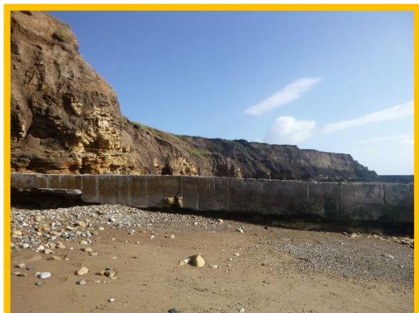
Undercutting to Ryhope Nook outfall. (Asset Ref. No. 121AB901B0804C03)
