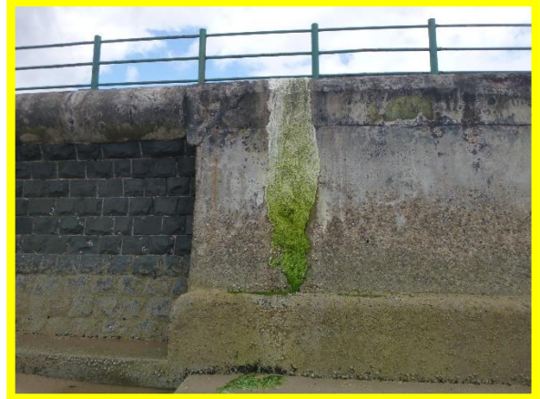
Damaged section of coping and chloride staining (Asset Ref. No. 121AB901B0604C01)
