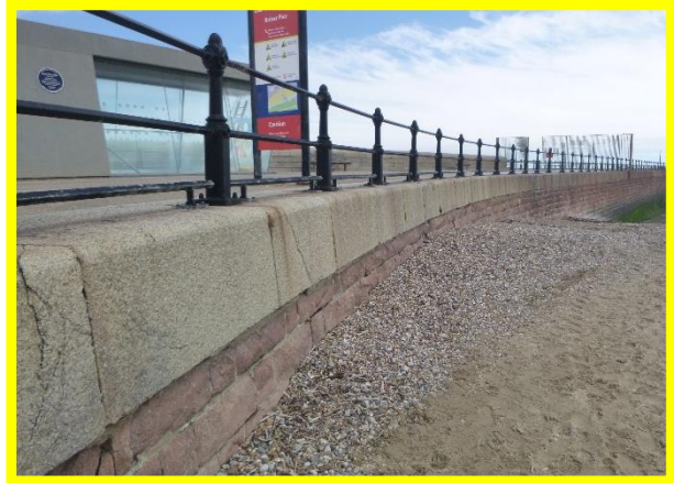
Masonry splash wall at southern root of pier – sections of damaged coping and weathered masonry. (Asset Ref. No. 121AB901B0702C05)
