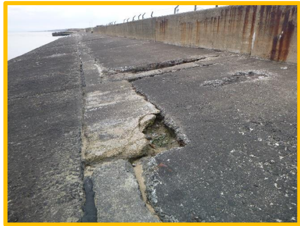
Various cracks and open joints to deck slab with past concrete repairs. (Asset Ref. No. 121AB901B0802C01)
