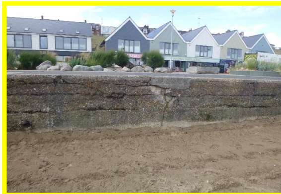
Patch repairs and horizontal cracks in concrete wall. (Asset Ref. No. 121AB901B0702C01)
