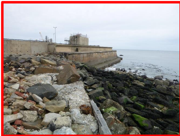
Scour hole at north end has been infilled with rock armour.. (Asset Ref. No. 121B901B0802C03)
