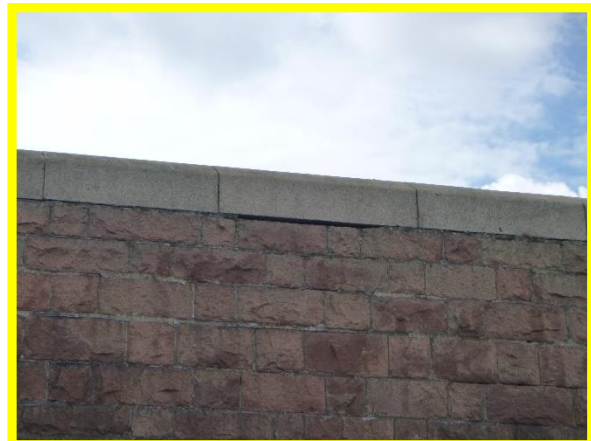
Roker Pier northern (outer) face, vertical cracks and open joints along coping (Asset Ref. No. 121AB901B0702C05)
