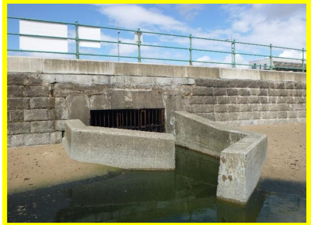
Repaired concrete coping above outfall structure in fair condition. (Asset Ref No. 121AB901B0603C02)
