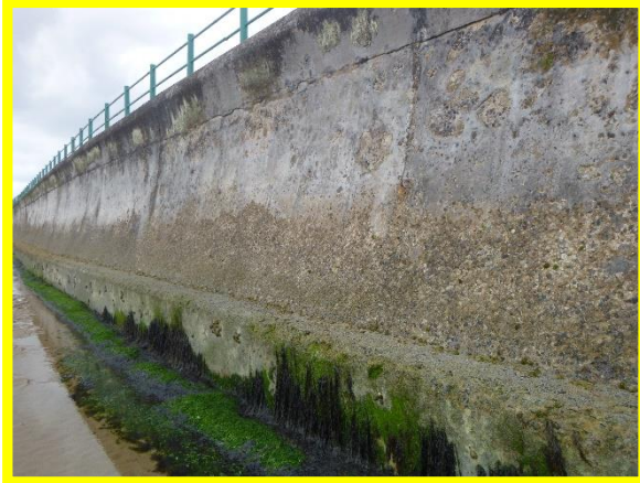
Beach levels marginally lower than 2020, spalling damage at crest and abrasion across wall face. (Asset Ref. No. 121AB901B0604C01)
