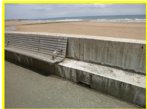
Rust staining and cracking in crest wall. (Asset Ref. No. 121AB901B0603C03)
