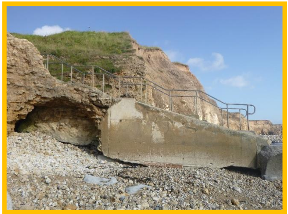
Access steps at Ryhope Village Dene in fair condition, although locally undercut. (Asset Ref. No. 121AB901B0804C02)
