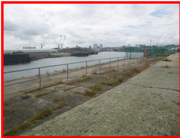
Cracked deck slab and splash wall with vegetation growth throughout. (Asset Ref. No. 121AB901B0702C03)
