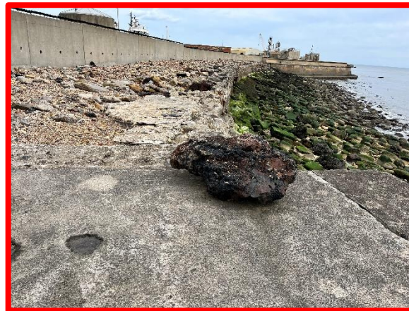
Unprotected crest apron and rear concrete boundary wall. (Asset Ref. No. 121B901B0802C03)
