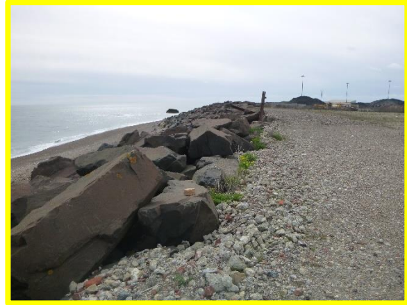
Uneven crest level of revetment. Embankment to rear has been reprofiled and is in good condition (Asset Ref. No.121AB901B0801C02)
