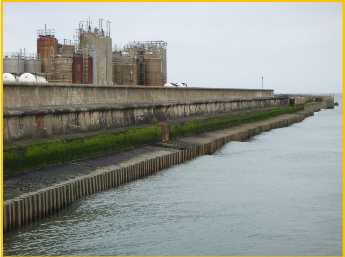
Spur Barrier wall in fair overall condition with evidence of localised damage throughout structure. (Asset Ref. No. 121AB901B0802C04)
