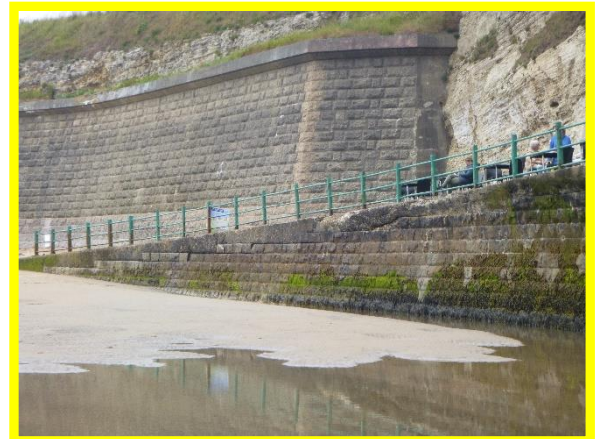
Damage to coping on ramp south of Parsons Rocks. (Asset Ref. No. 121AB901B0604C02)
