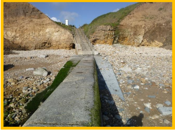
Access steps at Ryhope Village Dene in fair condition, although locally undercut. (Asset Ref. No. 121AB901B0804C02)
