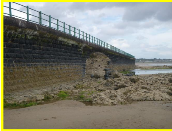
Remains of previous access steps breaking up onto foreshore. (Asset Ref. No. 121AB901B0604C02)
