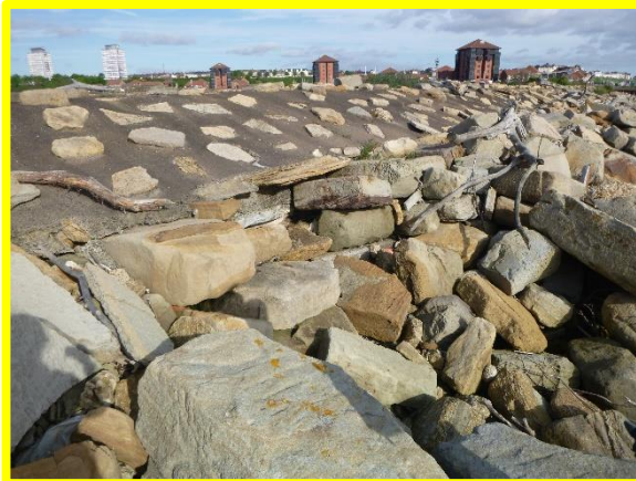
View of slumping at southern end of revetment (Asset Ref. No. 121AB901BO703C03)
