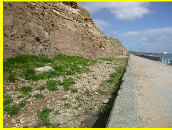
Localised gullying of slope to rear of seawall (Asset Ref. No. 121AB901B0803C02).
