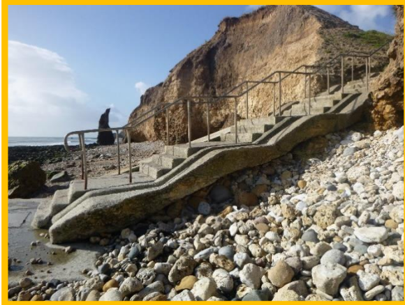
Access steps at Ryhope Village Dene in fair condition (Asset Ref. No. 121AB901B0804C02)
