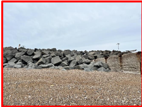
Derelict concrete groyne from north. (Asset Ref. No. 121AB901B0801C06)
