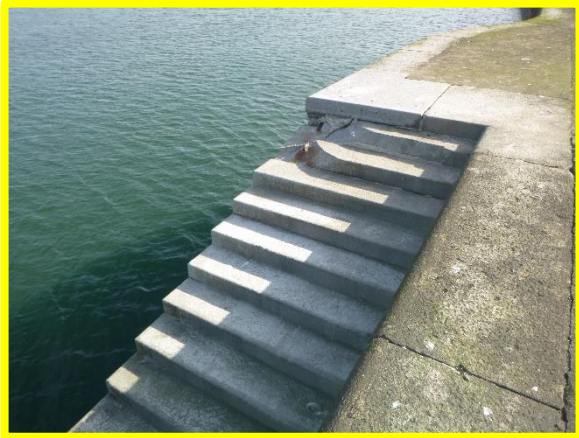
Damage to access steps. (Asset Ref. No. 121AB901B0703C01)
