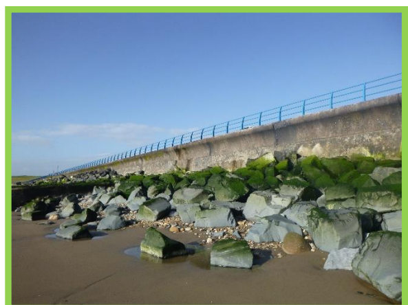
Movement of rock armour (Asset Ref. No. 121AB901B0803C02)
