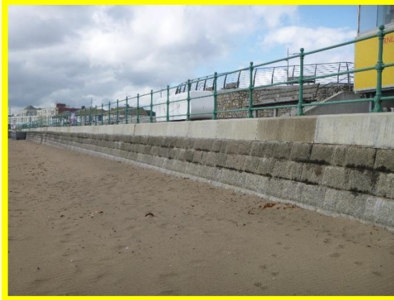
Repaired concrete coping above masonry seawall generally in good condition. (Asset Ref No. 121AB901B0603C02)
