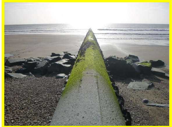
Concrete sewage outfall pipe in fair condition, heavily corroded / abraded at pile head. (Asset Ref. No. 121AB901B0803C02)
