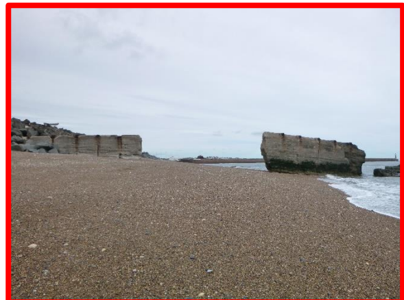
Derelict concrete groyne from south. (Asset Ref. No. 121AB901B0801C01)
