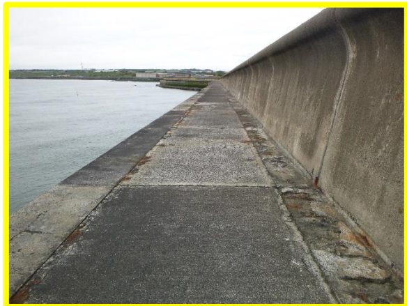
Cracking and spalling of upper sea wall. (Asset Ref. No. 121AB901B0802C04)
