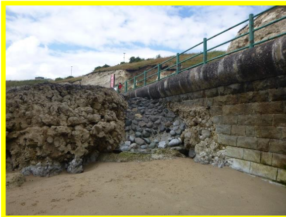
Eroded limestone outcrop void beneath promenade at south of Parsons Rocks. (Asset Ref. No. 121AB901B0604C02)
