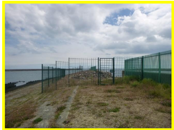
Fencing detached locally enabling access by public to unsafe structure. (Asset Ref. No. 121AB901B0702C03)
