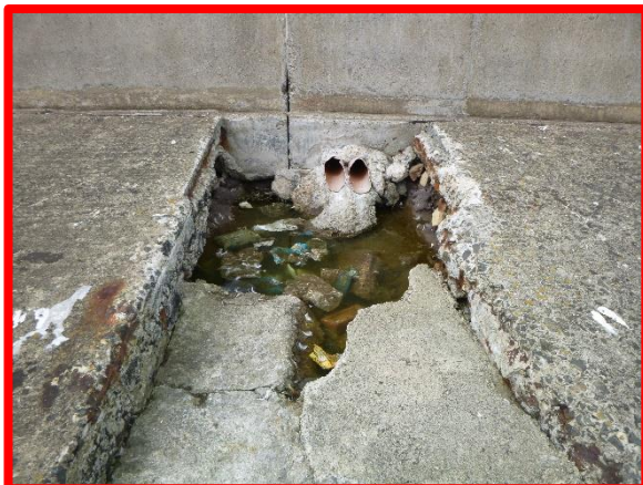
Example of damaged deck slab at outfall drain leading to washout of infill material. (Asset Ref. No. 121AB901B0802C01)
