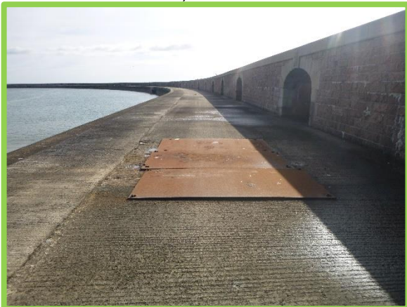
Steel sheet covering void reported in 2018. (Asset Ref. No. 121AB901B0703C01)
