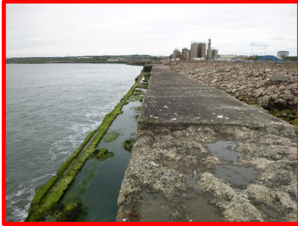
Extensive damage to concrete apron on seaward face of structure. (Asset Ref. 121AB901B0802C05)
