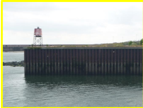
View on sheet pile river navigation wall, noted previously with staining indicating microbial induced corrosion (MIC) reducing structural capacity (Asset Ref. No. 121AB901BO703C03)
