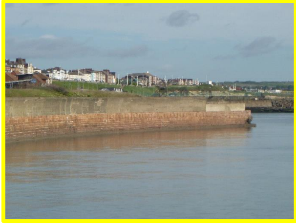
Masonry wall in fair condition except for missing blocks at North end. (Asset Ref. No. 121AB901BO703C02)
