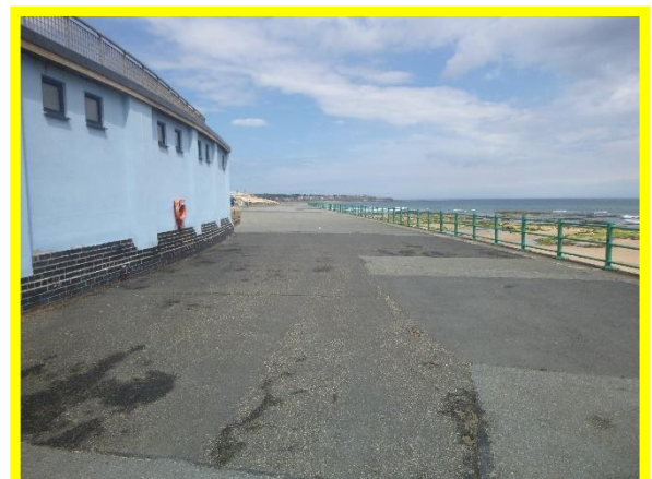
Recently infilled voids in grouted revetment (Asset Ref. No. 121AB901B0604C02)
