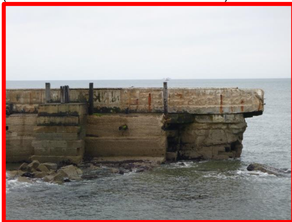
Nose of pier undercut. (Asset Ref. No. 121B901B0801C04)
