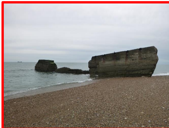
Derelict concrete groyne from north. (Asset Ref. No. 121AB901B0801C01)
