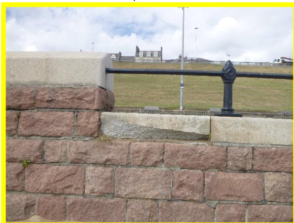
Damage to coping stone, similar to 2020. (Asset Ref. No. 121AB901B0605C02)
