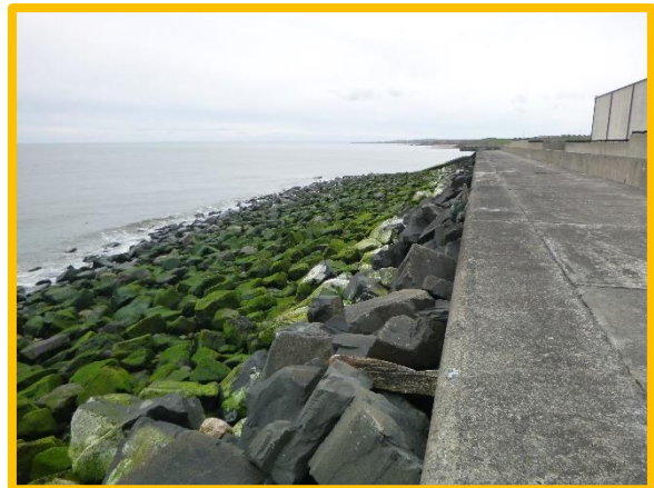
Steep, uneven rock armour profile. (Asset Ref. No. 121AB901B0802C02)
