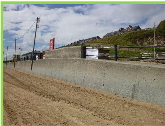
Low concrete encased wall at Marine Walk in fair to good condition. (Asset Ref. No. 121AB901B0605C02)
