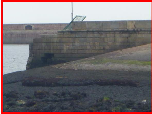
Missing blocks at seaward end of Old North Pier. (Asset Ref. No. 121AB901B0702C03)
