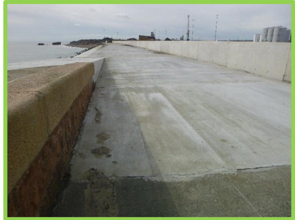
Deck slab repaired and new precast splash wall constructed. (Asset Ref. No. B901B0801C03)
