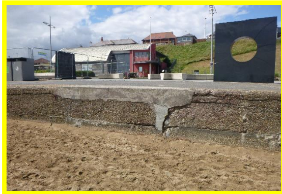
Patch repairs and horizontal cracks in concrete wall. (Asset Ref. No. 121AB901B0702C01)
