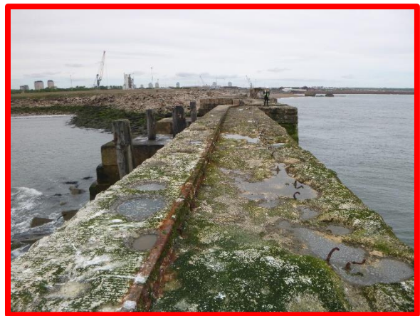
Heavily abraded deck. (Asset Ref. No. 121B901B0801C04)
