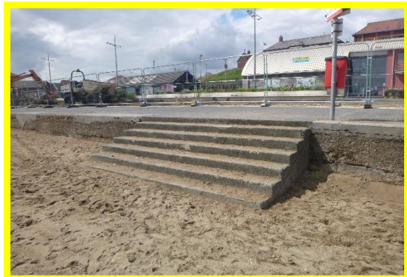
Example of spalling between horizontal cracking (Asset Ref. No. 121AB901B0702C01)
