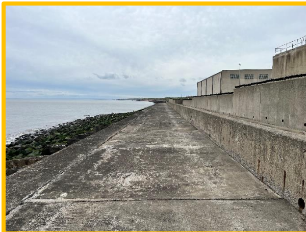
Abrasion and cracking of deck slab. (Asset Ref. No. 121AB901B0802C02)
