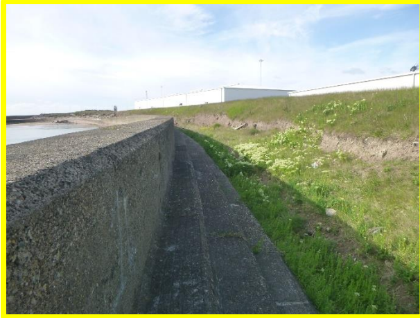
Extensive crest and rear embankment damage due to wave overtopping. (Asset Ref. No. 121AB901BO703C02)
