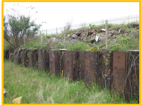
Heavily corroded sheet pile wall (Asset Ref. No. 121AB901B0802C07).
