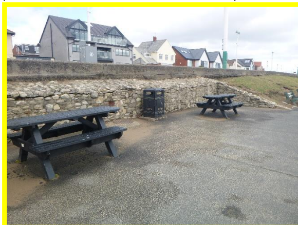
Lateral crack along rear of revetment at picnic area (Asset Ref No. 121AB901B0603C01)
