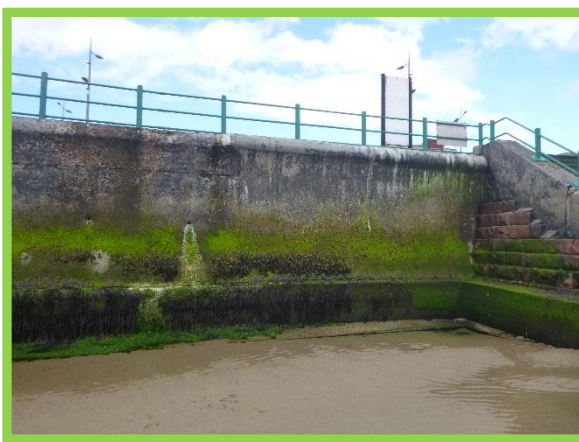
Recently constructed seawall infill section adjacent to steps at Seaburn Terrace (Asset Ref. No. 121AB901B0603C03)
